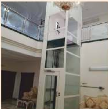
Hydraulic Home Lift
